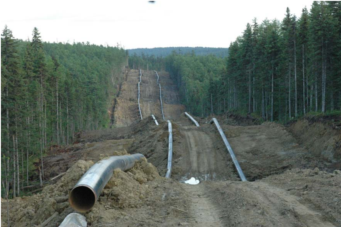
Pipelines of Sakhalin 2 project near the nest sites of the Steller's Sea Eagle.
