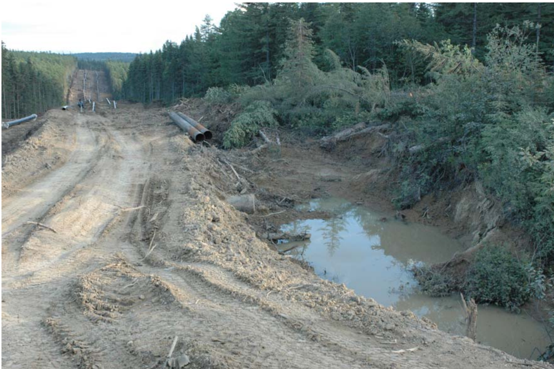
Pipelines will cross over more than 1000 rivers. The destruction of the source of eagle food (salmon) will easily happen.
